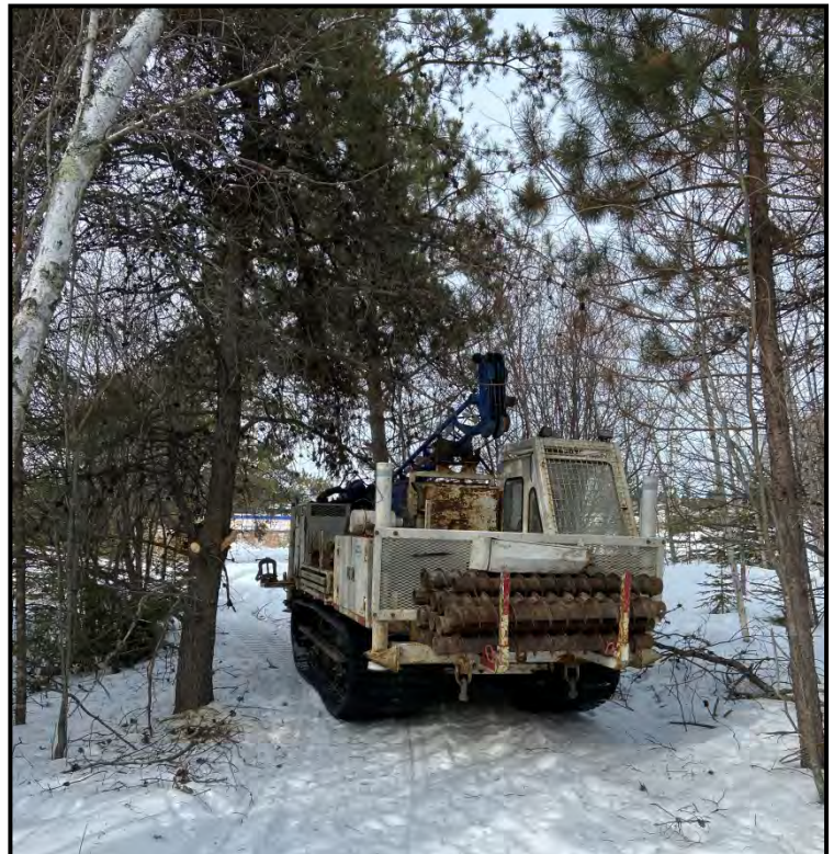
PHOTOGRAPH #4: Mobilizing in the forested area in the southeast portion of the Site.
